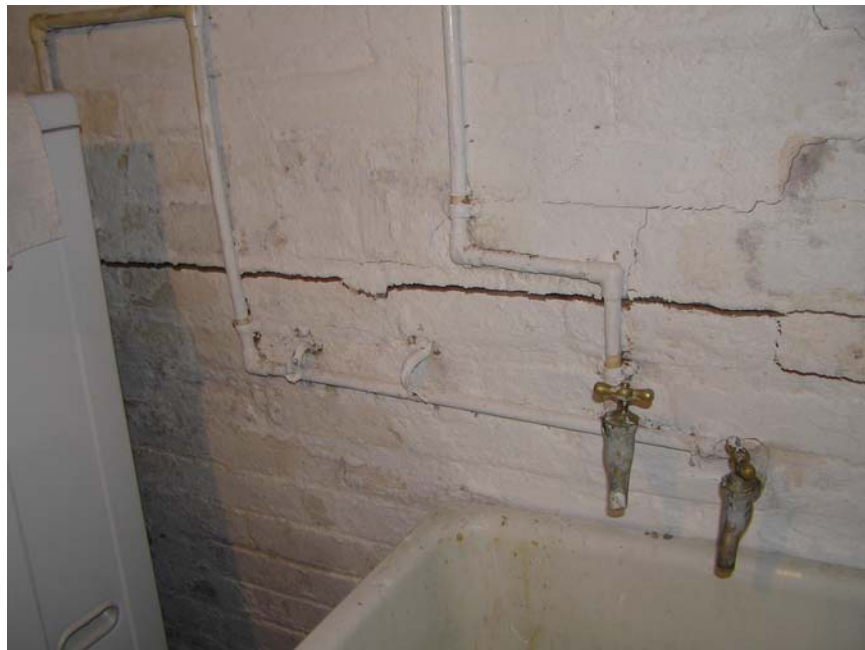
Figure 4 Interior face of wall exhibits staining, peeling paint, blistering of paint, mineral deposits, and repeated paint coverage.
