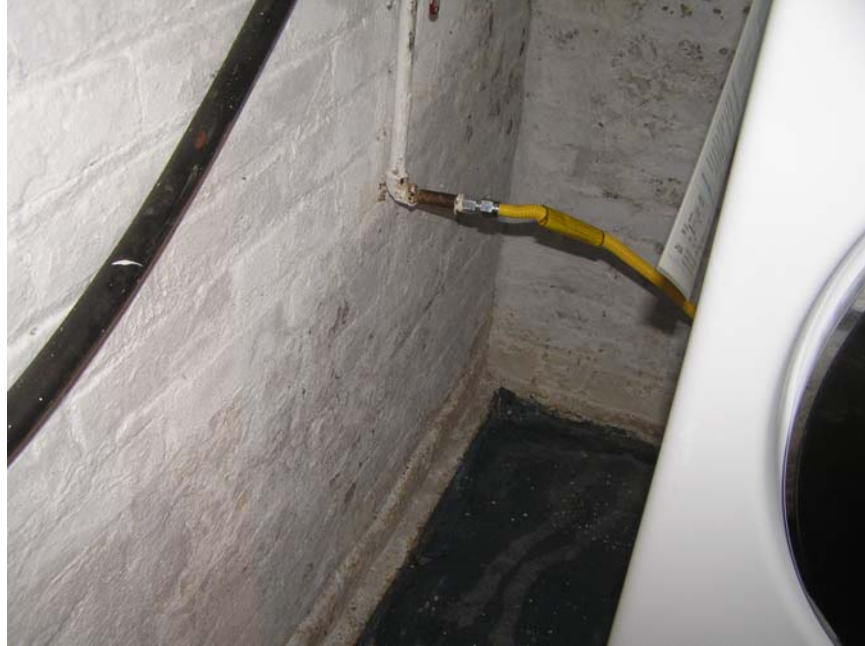
Figure 3 Interior face of wall exhibits staining, peeling paint, blistering of paint, mineral deposits, and repeated paint coverage.
