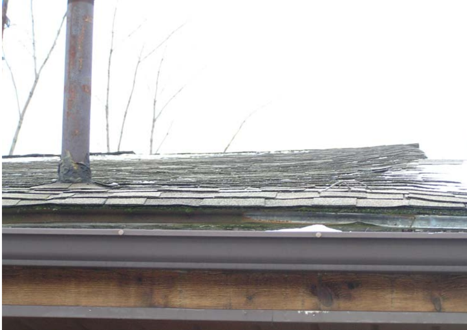
Figure 8 Roof sags from eave to ridge.
