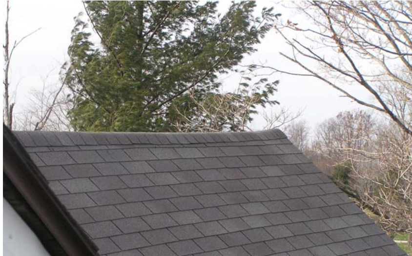
Figure 7 Shingle exposure varies exhibiting sag in roof.
