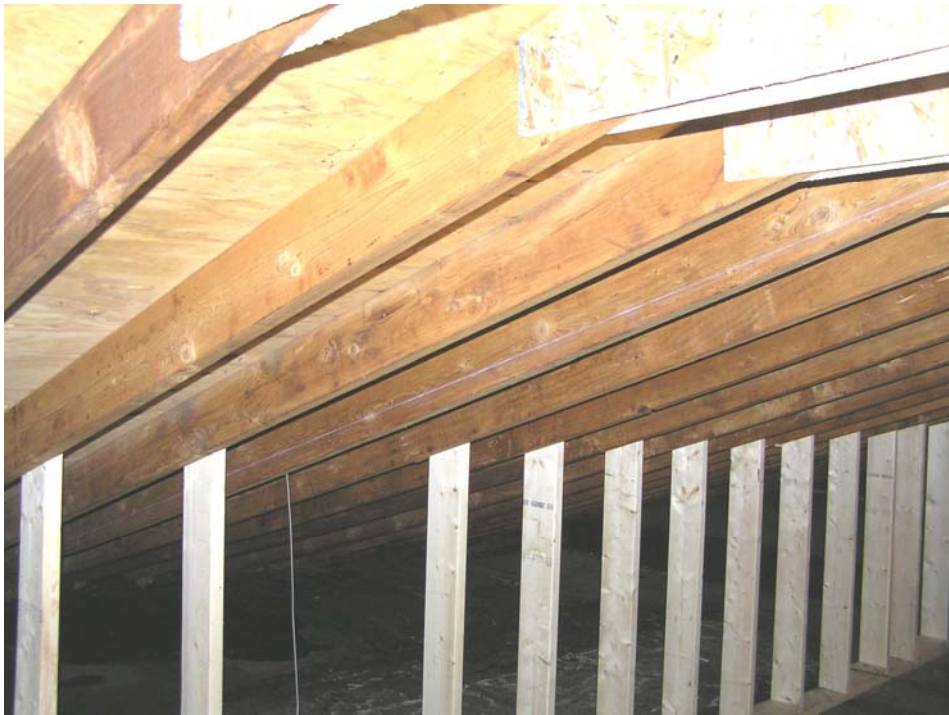
Figure 9 Chalk line on side of rafter shows amount of sag.
