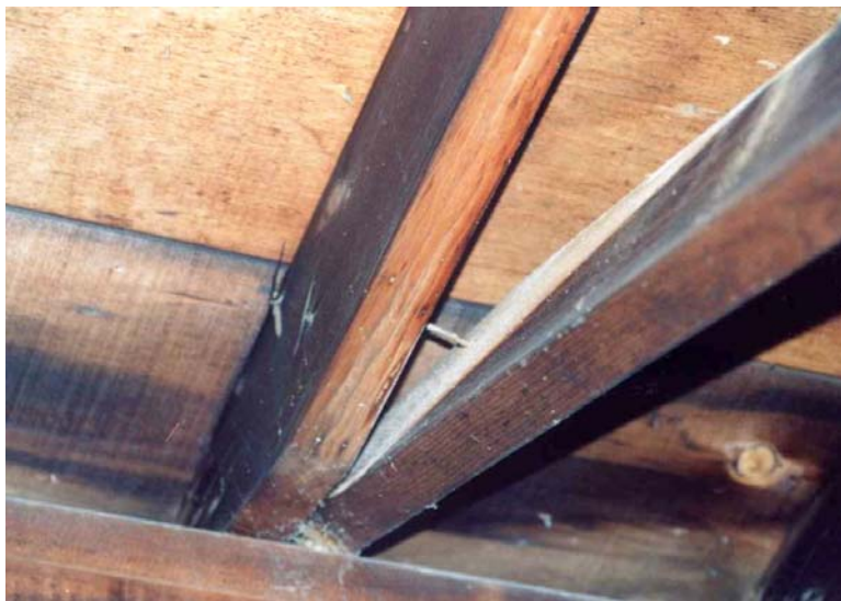
Figure 6 Ceiling tie fastened with one nail pulls away.
