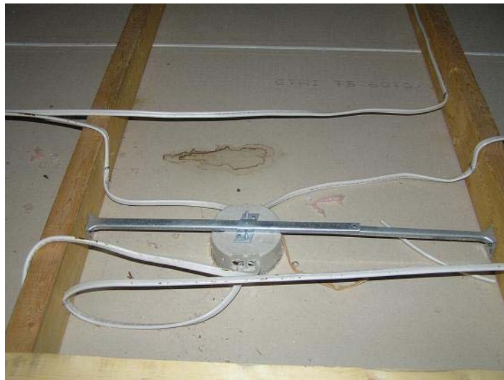
Figure 7 Moisture stain on top side of ceiling. Note multiple rings.
