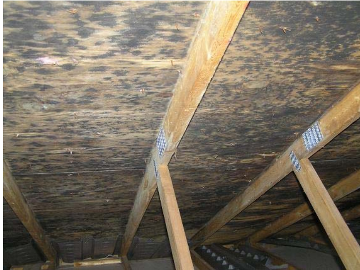
Figure 4 Widespread mold growth on underside of roof deck.
