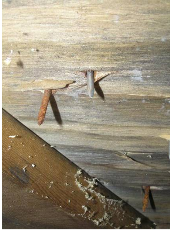
Figure 8 Corroded nails and clean nails present in the attic space.
