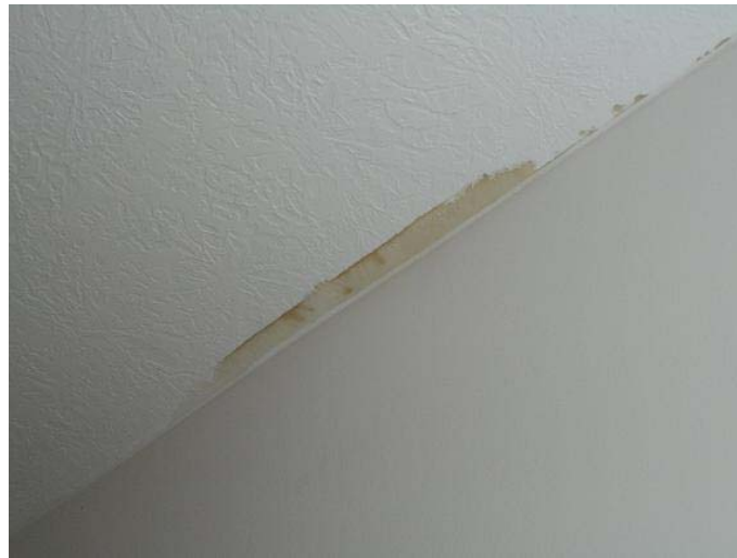
Figure 2 Tea colored staining on ceiling near the exterior wall.
