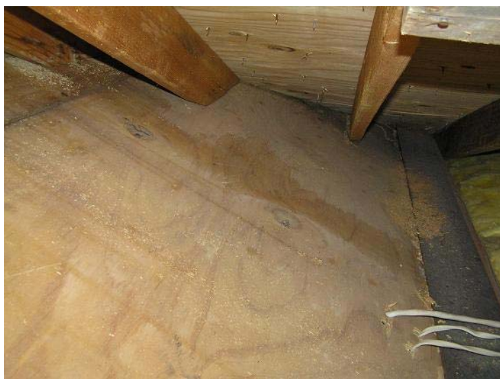
Figure 3 Roof leak at a valley.
