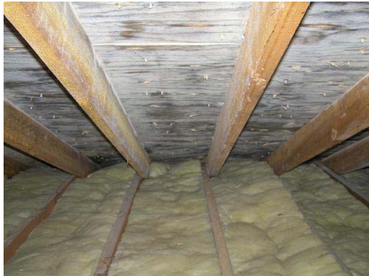
Figure 6 ventilation from eave restricted by insulation tight to roof deck.
