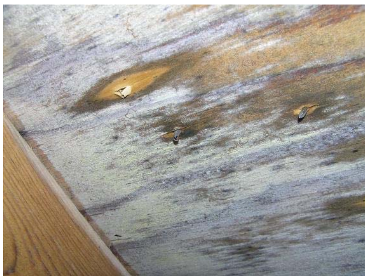
Figure 10 Roof deck clear at hole for removed galvanized roofing nail. Roof deck is mold covered around newer roofing nails.
