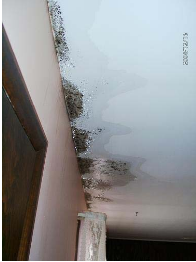
Figure 1 Mold growth and water droplets on ceiling.
