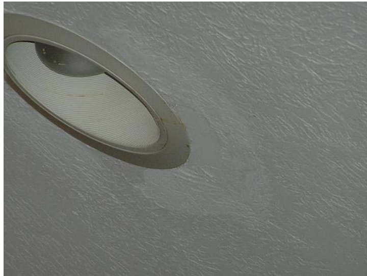
Figure 9 Previous paint coverage at area of moisture staining.
